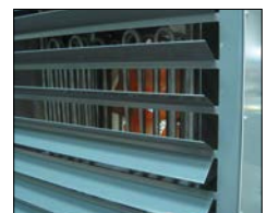
Detalle deflectores. View of deflectors.
